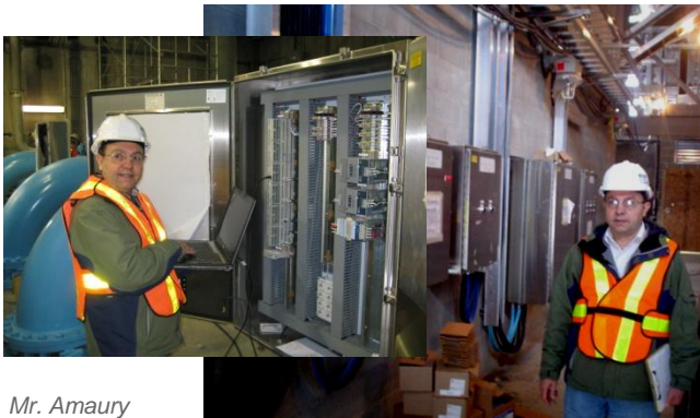
Mr. Amaury Pereira, P.Eng RTS' Electrical Control Panel Specialist at the Control Room
