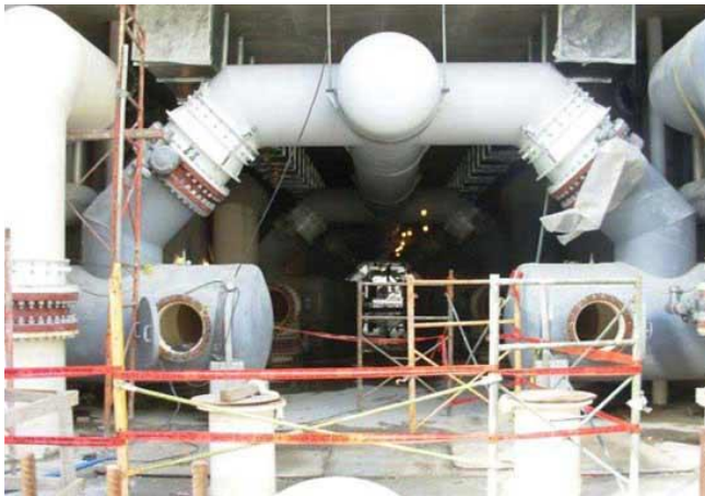
The filtration pipe gallery. The project was largely driven by the need to reduce turbidity
