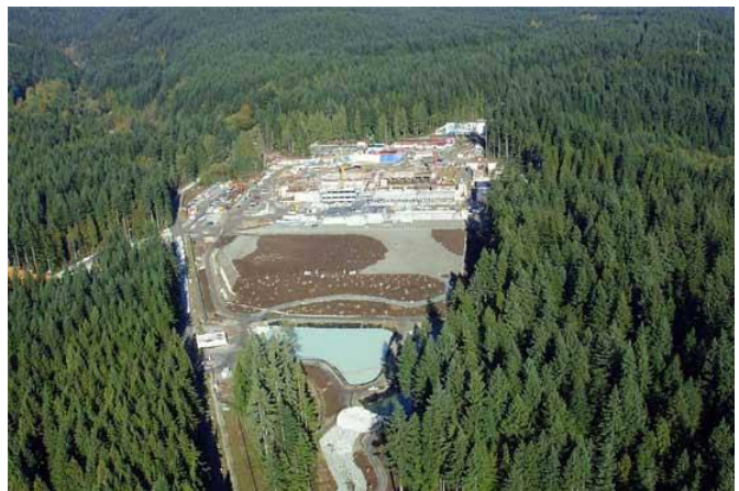
Aerial view of the filtration plant; it occupies a site of around 8 hectares, located in the Lower Seymour Conservation Reserve.
